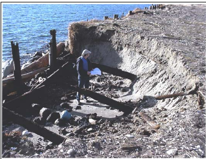
Breakwater damage from Thanksgiving Storm
