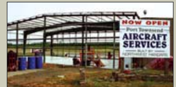
Port Townsend Aircraft Services is rebuilding at the airport after a fire.
