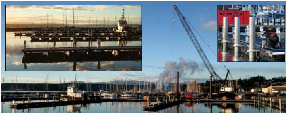
Pile-driving for A/B Dock is 60% complete and all but one of the lateral docks are afloat in these Dec. 10 photos; the finger floats have yet to be installed. A worker thermal-welds pipe for the fire suppression system.
