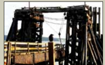
Quincy Street Dock shortly before winter storm repairs were made.
