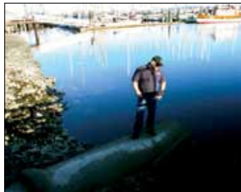
Port Environmental Compliance Officer Khile stands atop one of the Yard's two stormwater outfalls.
