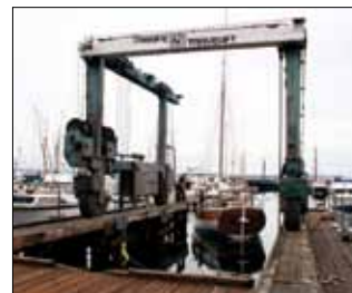
Construction of a new 75-ton Travelift pier begins this fall. It is used in 1,500 lift operations annually.
